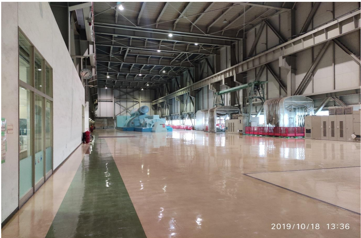
Reihoku: Turbine Floor
